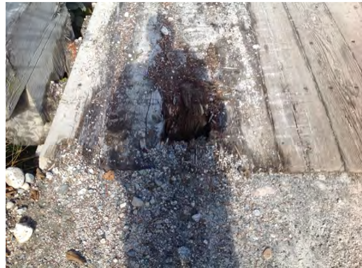
holes starting to form in deck
