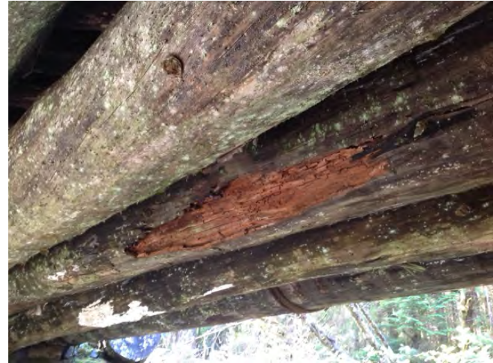
log stringer condition
